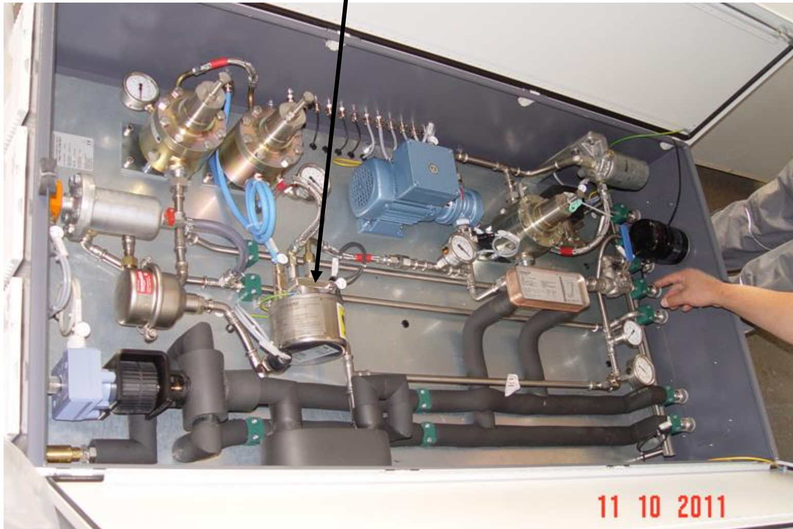
Coriolis Fuel Flow Meter in Fuel Conditioning Cabinet
